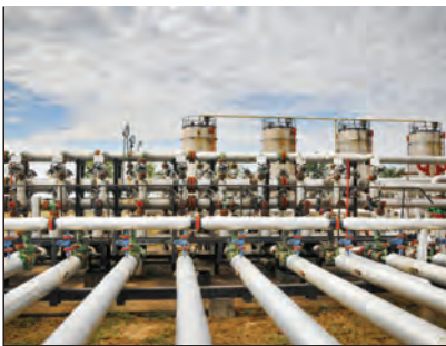
Natural Gas Fueling Pipeline
