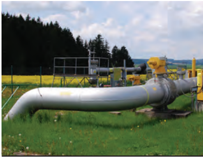
Natural Gas Pipeline
