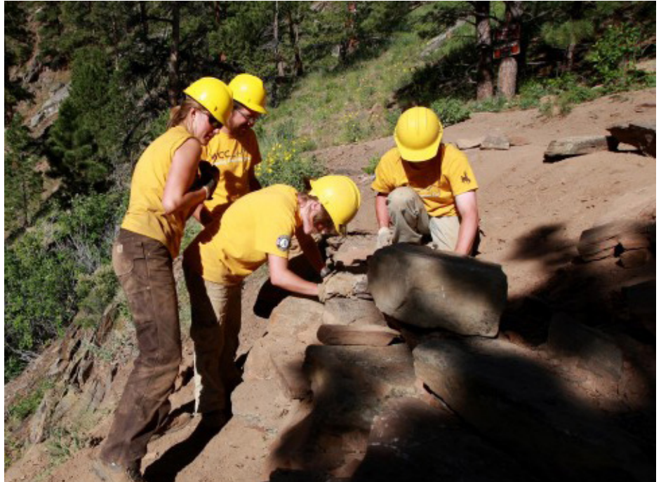
From left, Wyoming Conservation Corps members Anna Kramer, Andrew Mittelstadt, Lee Rogers and Phineas Peake rebuild a stone retaining wall along the Bridle Trail on Casper Mountain. An eight-person WCC crew is spending 10 days making improvements and repairs to the trail. Alan Rogers, Star Tribune
